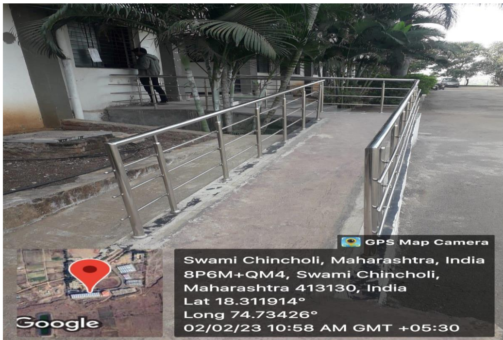
Geo-tagged photograph of Ramp for Disabled Friendly Person.
