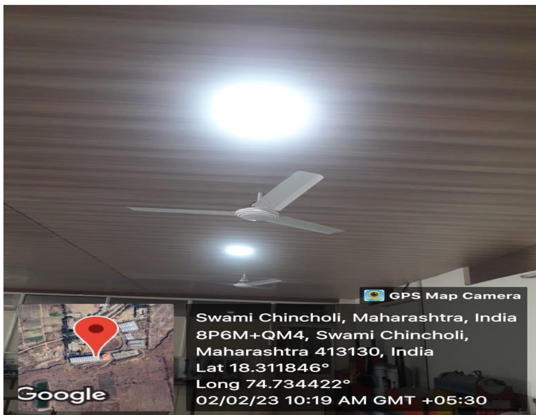
Geo-tagged photograph of use of LED Bulbs in Basic Mechanical Lab.
