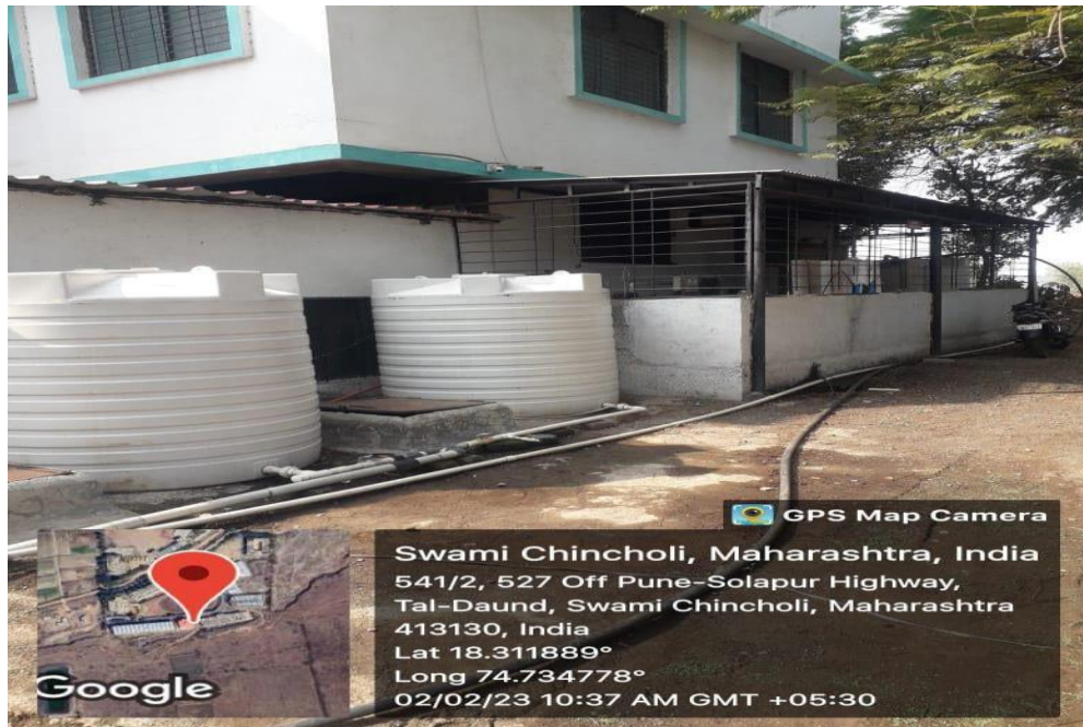
Geo-tagged photograph of Water Filter Plant Available in Campus.
