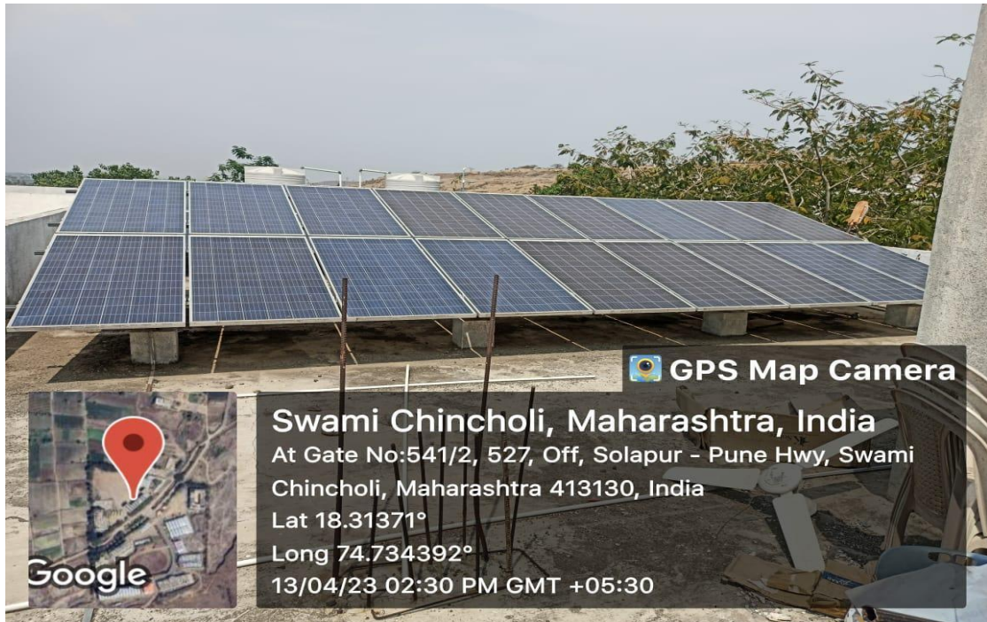
Geo-tagged photograph of Solar Power Plant installed on roof of Dattakala Campus.
