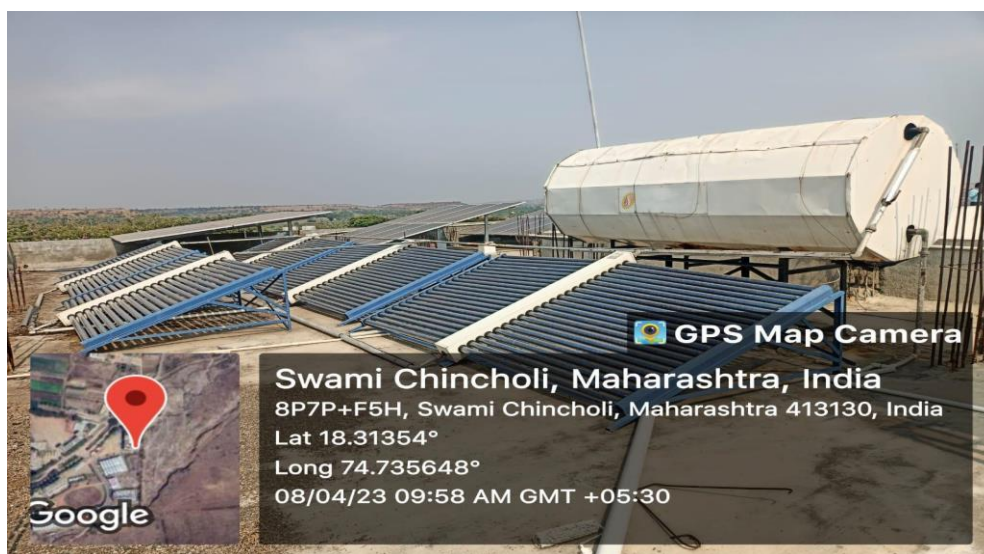
Geo-tagged photograph of Solar water heating system installed on roof of girl's hostel.
