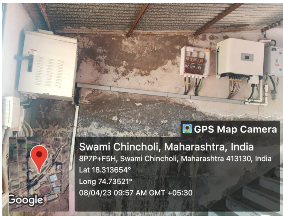
Geo-tagged photograph of Invertors to convers DC to AC on roof of girl's hostel.
