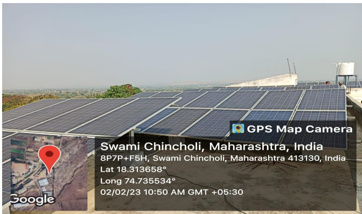
Geo-tagged photograph of Solar Power Plant installed on roof of girls hostel.
