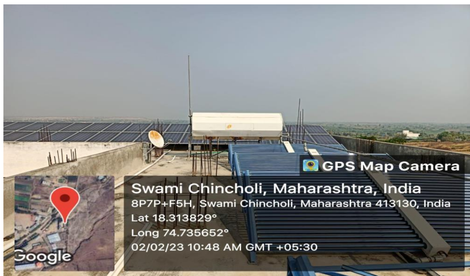
Geo-tagged photograph of Solar water heating system installed on roof of girl's hostel.
