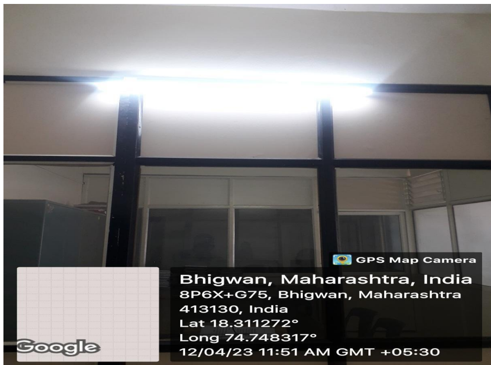
Geo-tagged photograph of use of LED tubes in exam room on first floor.
