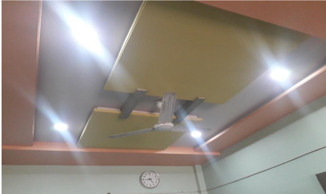
Photograph of use of LED Bulbs in Principals Cabin.
