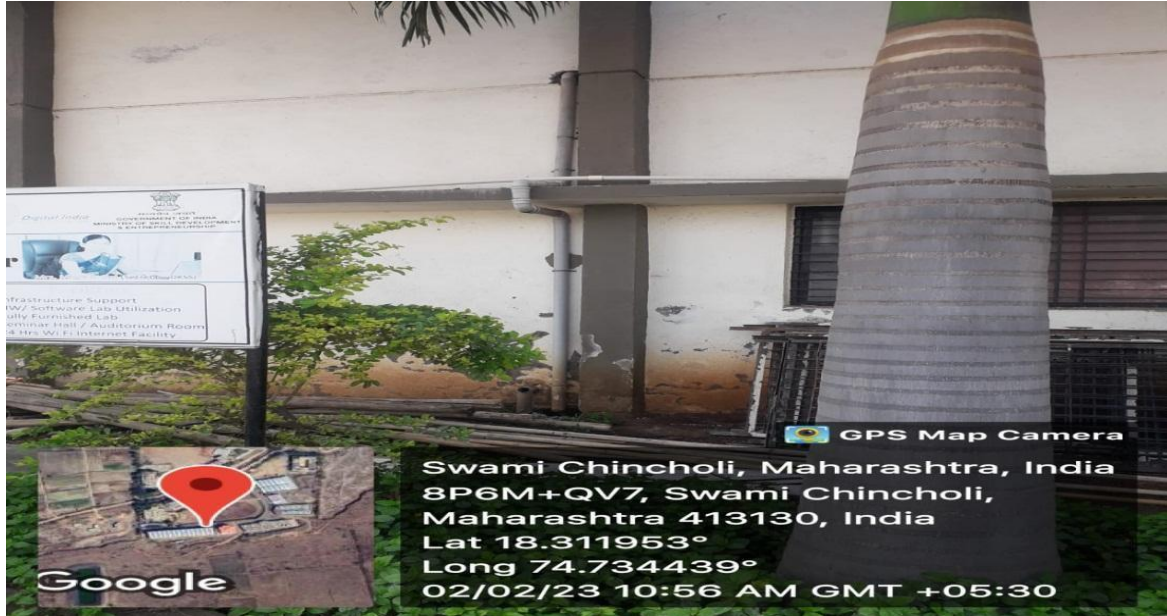
Geo-tagged photograph of Pipes for Collecting Rain Water.
