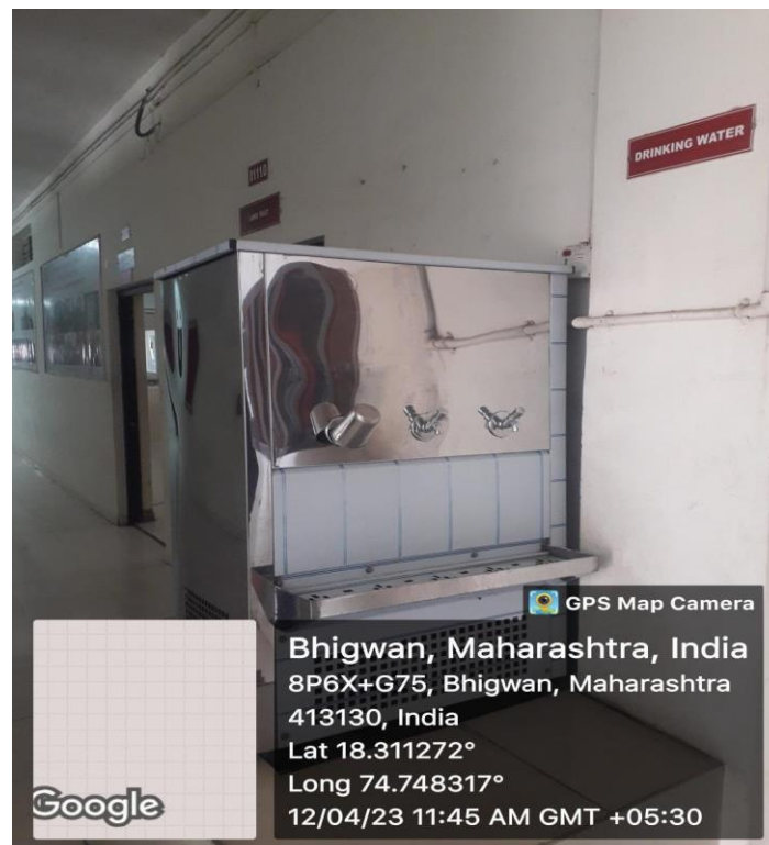
Geo-tagged photograph of Water Filter Tank for Drinking Water First Floor.
