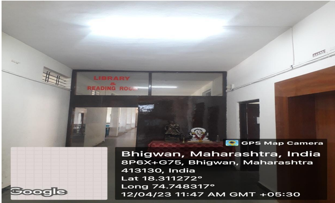
Geo-tagged photograph of use of LED tubes in the library on the ground floor.
