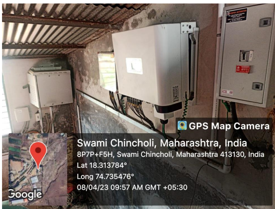
Geo-tagged photograph of Invertors to convers DC to AC on roof of girl's hostel.
