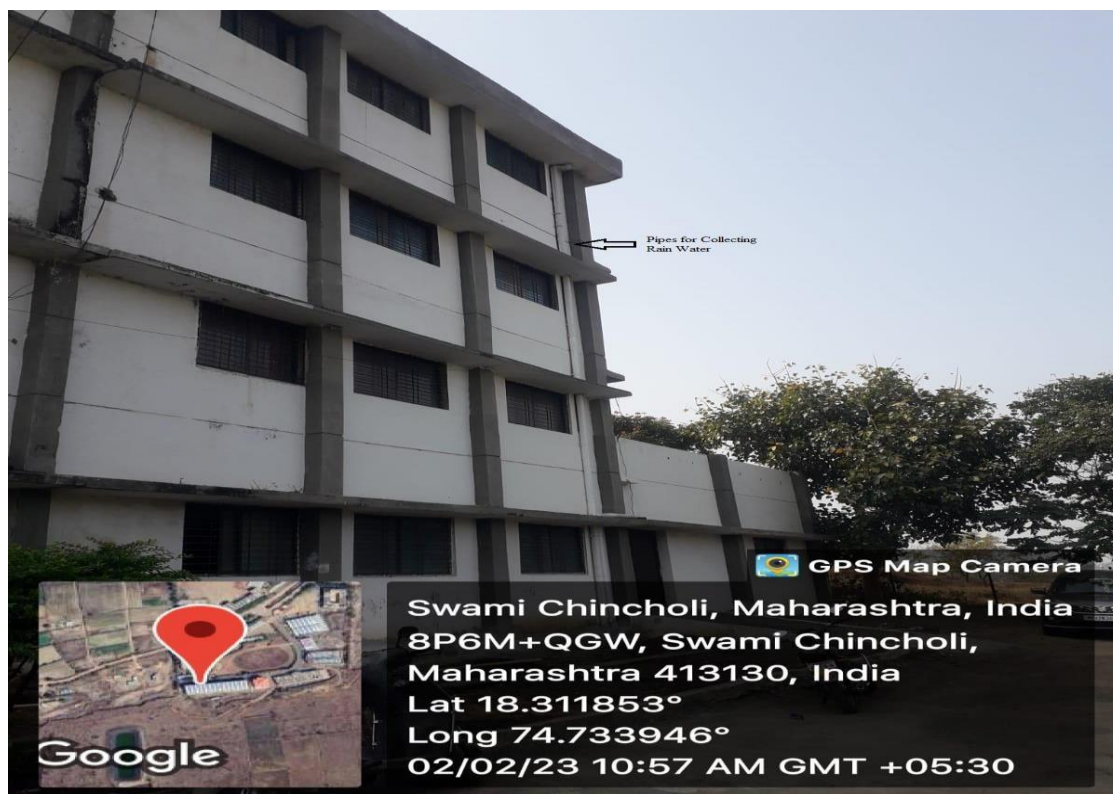
Geo-tagged photograph of Pipes for Collecting Rain Water.
